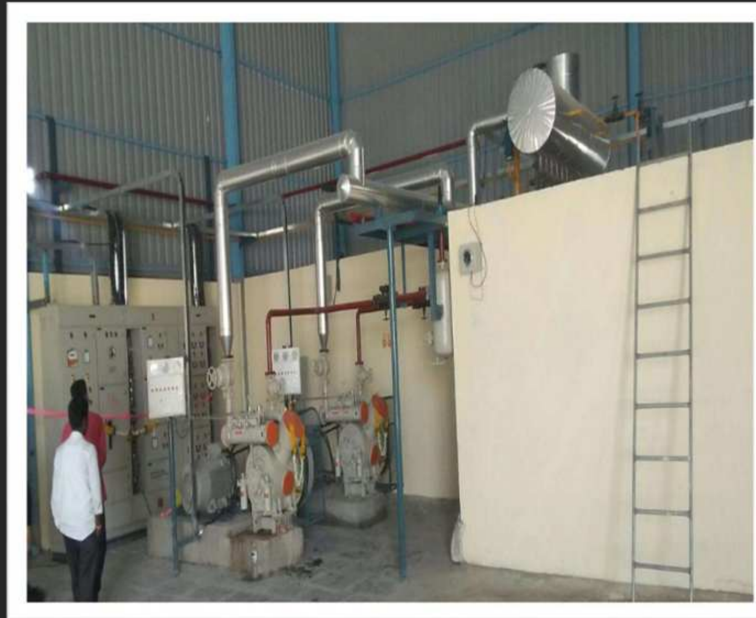
AMMONIA ICE BANK TANK
