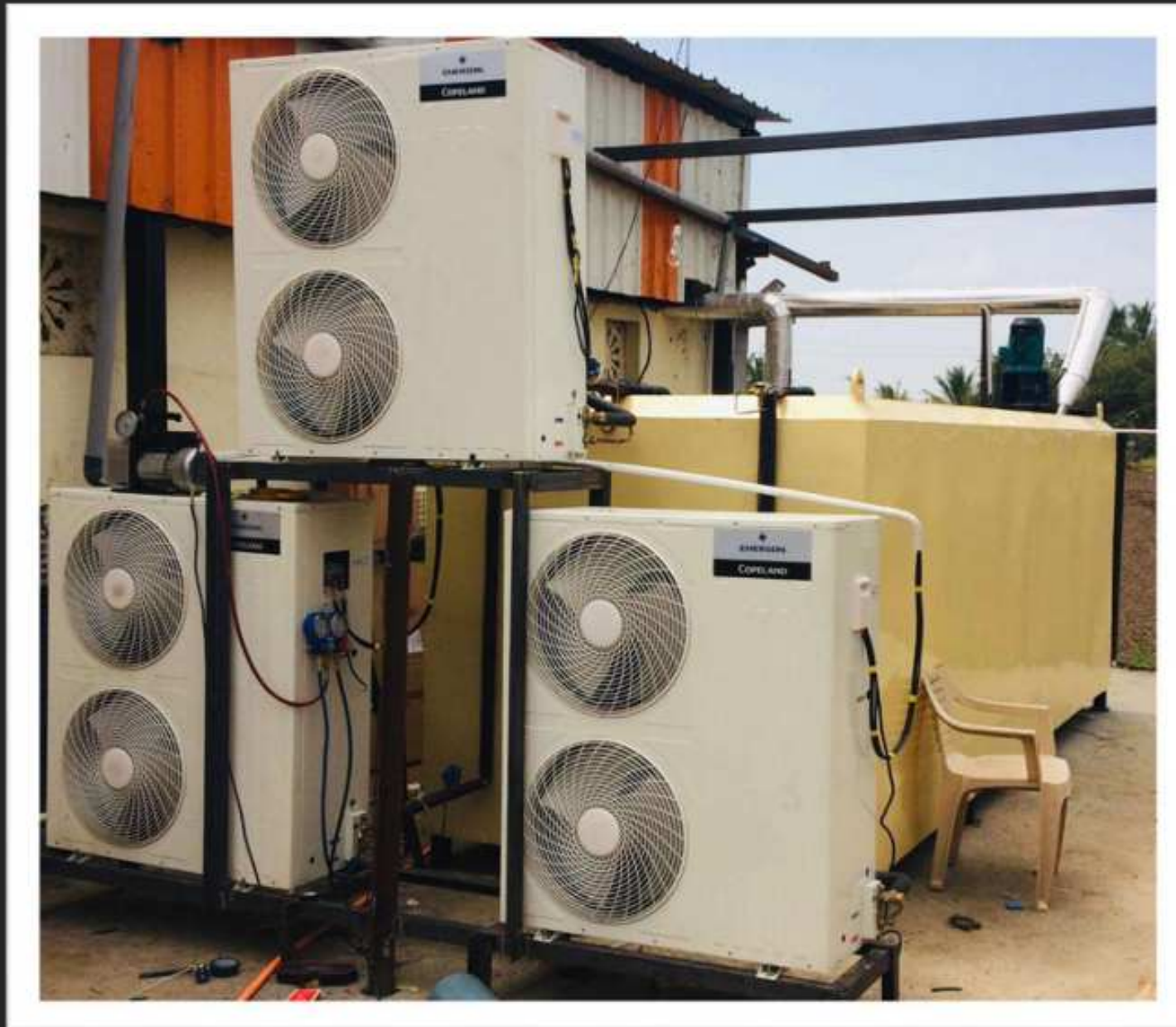
FREON ICE BANK TANK
