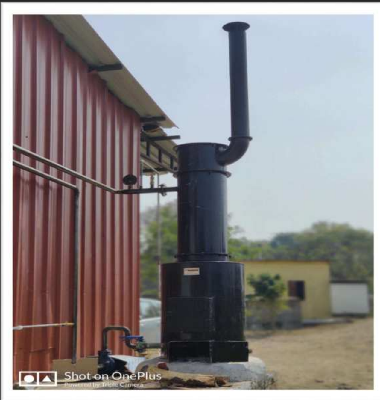
HOT WATER BOILER
