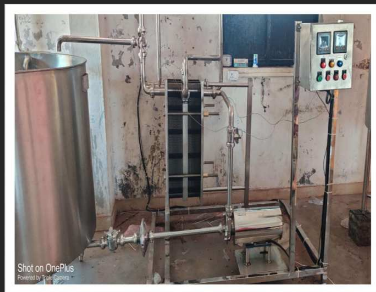
Double Stage P.H.E ( Skid mounted)
