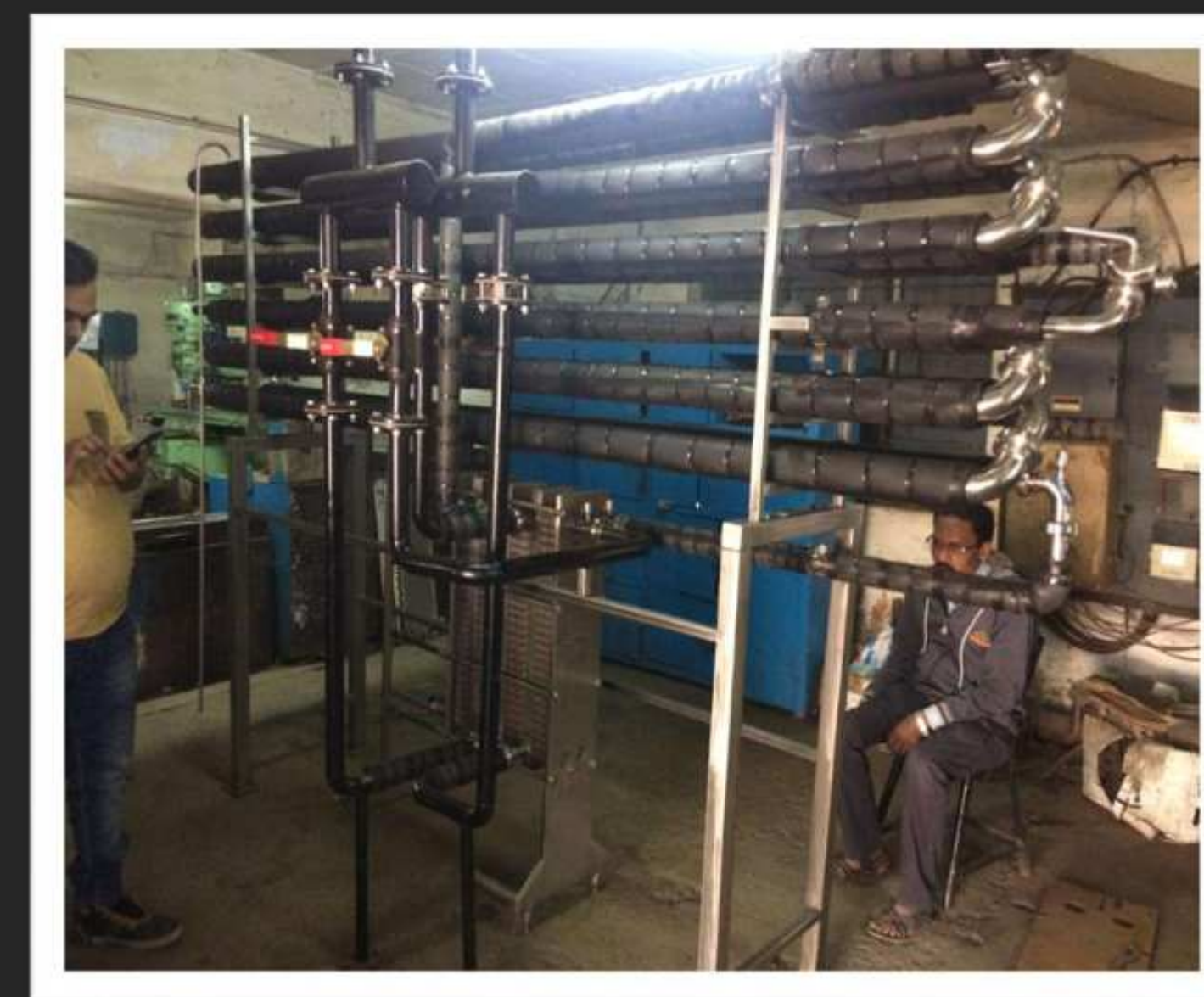
Plate Heat Exchanger (Paneer / Curd)
